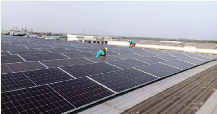
Solar Panels on rooftops of Market Buidling (1)
