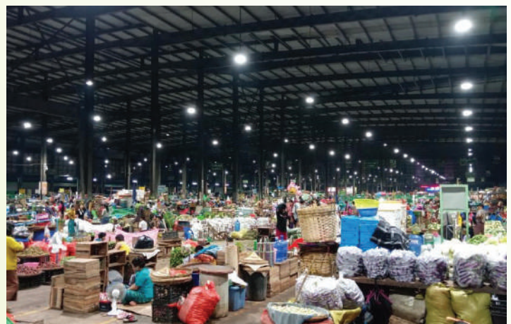
LED Lighting around Market Building
